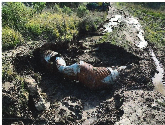
Damaged CMP culvert Access road, sewer trunk line
