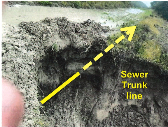
Wash-out Offsite 10-inch sewer trunk line
