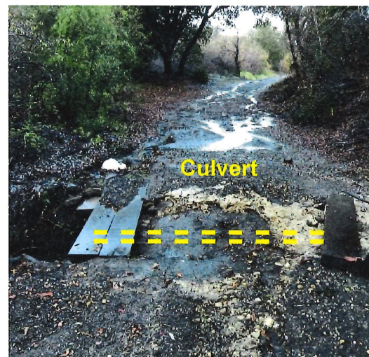
Damaged CMP culvert Access road, Lift Station #1
